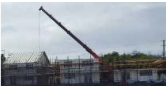
Fig. 2: Shows modules as they are being installed, two on the ground floor to the right, 4 modules in the centre and all 6 modules complete on the left
